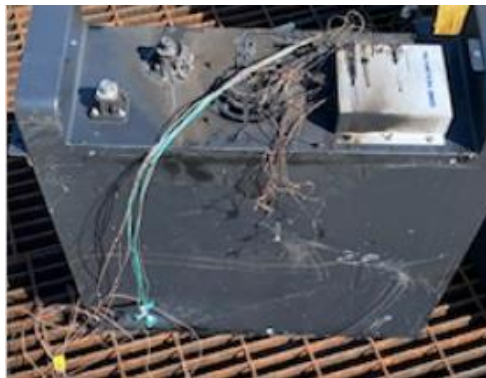
Figure 2 Damaged power storage unit battery
